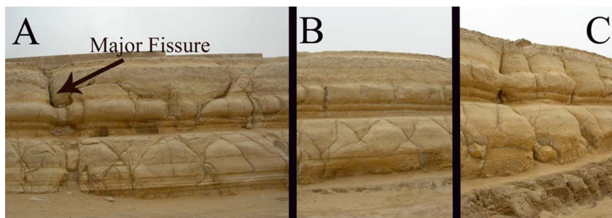
Figure 4. Sequence of three photographs of the southern enclosure wall, indicating significant differences in erosion. A: Intense erosion near the major fissure. B: A considerable decrease in erosion a bit further west. Also notice the almost complete lack of gullying on the upper layers. C: Noticeably increased erosion at the most western end of the southern enclosure wall. Photographs courtesy John Wall.
